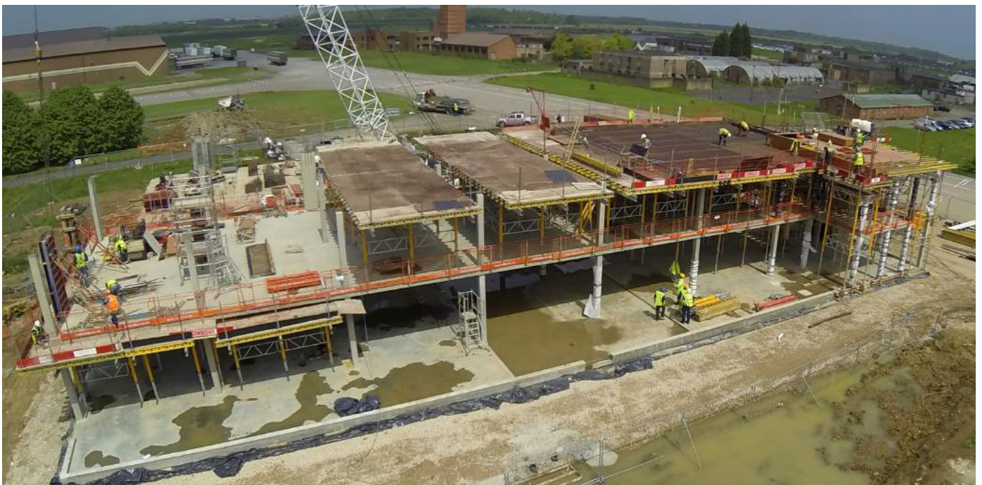
Peri-deck system + BAMTEC reinforcement to flat slab structure (image by Jason Hawkes)
