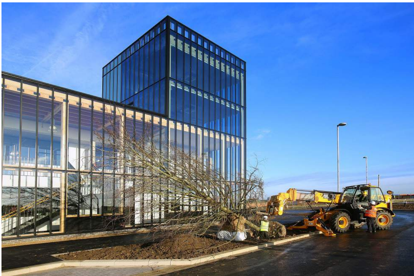
Erection of lime trees on the main boulevard (image courtesy of Urban + Civic)
